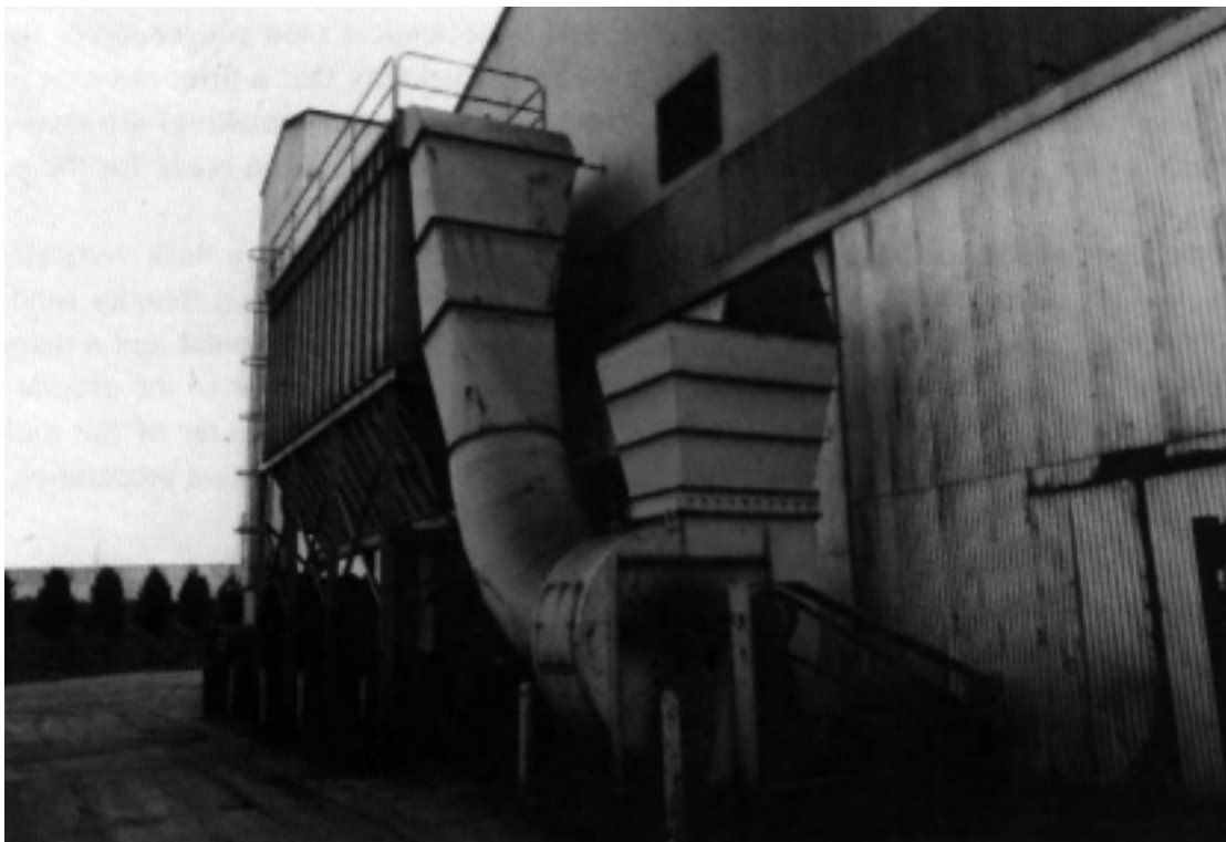
FIG. 5 — Exterior View of a Cupola with Air Pollution Control Equipment
