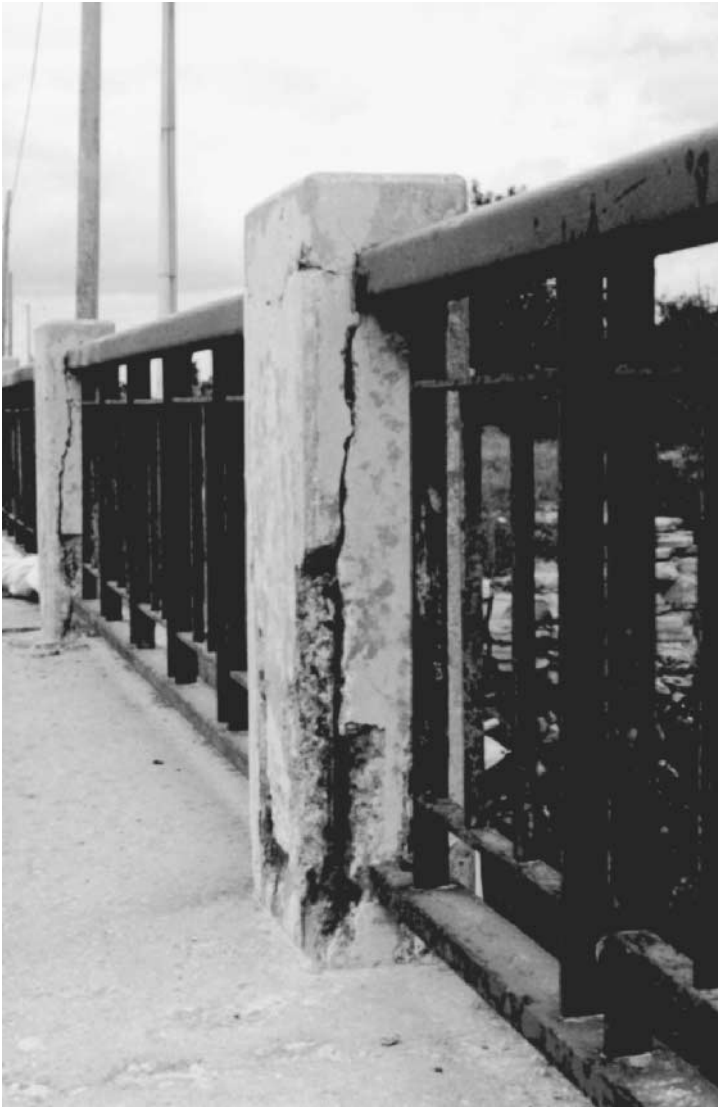
Figure 2.28 Concrete degradation caused by rebar corrosion damage near Kingston, Ontario. This bridge underwent extensive rehabilitation shortly after this picture was taken.
