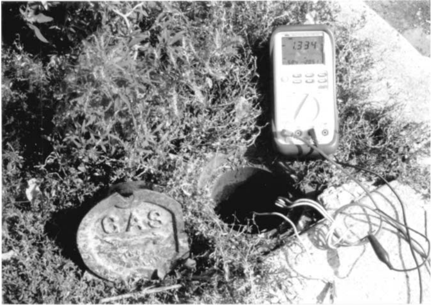
Figure 11.6 Ground-level test station used in urban areas.
