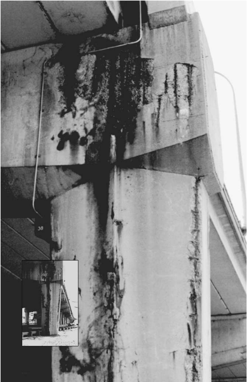
Figure 2.27 Concrete degradation caused by rebar corrosion damage in a highway structure in downtown Toronto, Ontario. Extensive repair work was underway on this structure at the time the picture was taken. The annual maintenance costs for this structure were recently reported at around $18 million.
