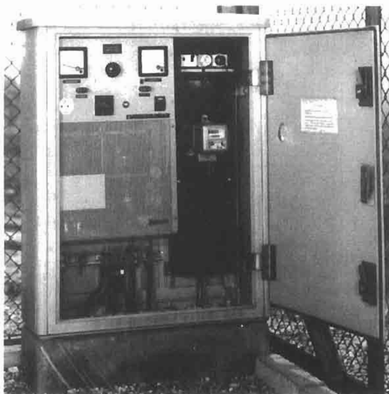
Fig. 8-2 Impressed current unit in a plastic housing with a meter panel.
