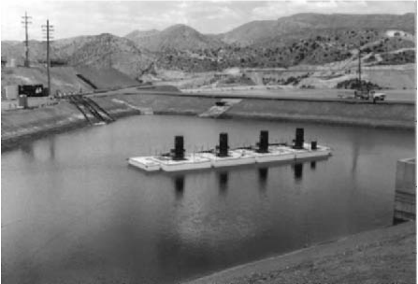
FIGURE 5 An installation of four floats with top inlet cantilevered shaft pumps (Hazleton Pumps, Inc.)
