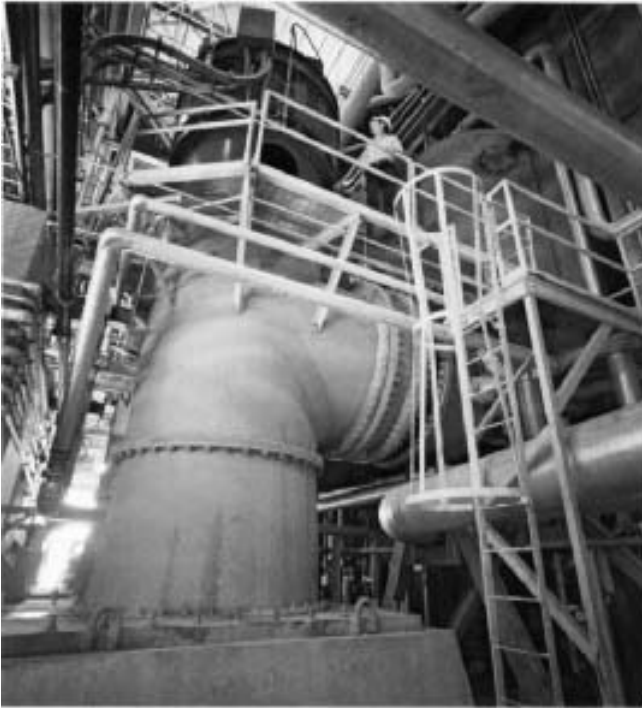
FIGURE 112 Vertical propeller pump installed (Flowsolve Corporation)
